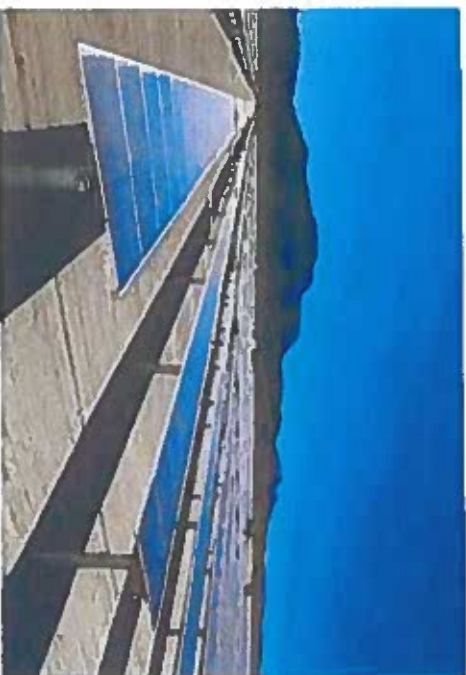
Mountain View Solar Project in Clark County, Nevada
