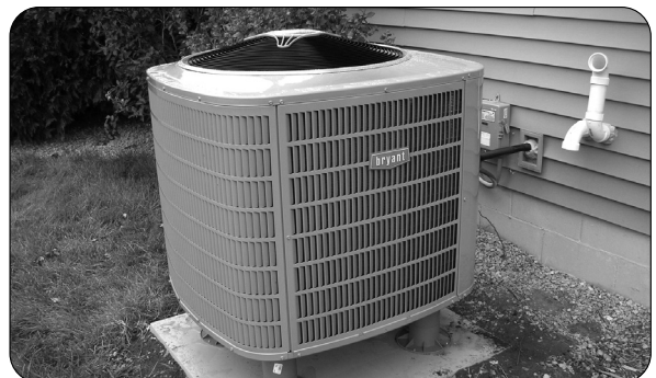
AIR CONDITIONING SYSTEM
