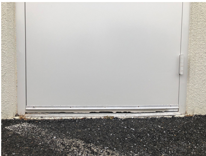
DOOR WITH A WORN OUT DOOR SWEEP
