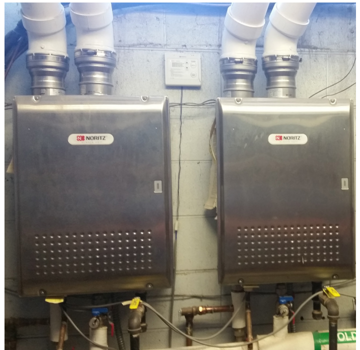
Tankless Water Heater for the School
