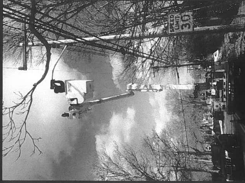
LED streetlight retrofit in Brewster
